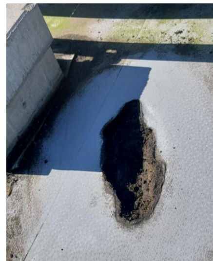
Figure 2 – Charred area on the roof surface caused by direct current arcing related to a faulty component of a BAPV system. The component was not located in the cavity between the roof surface and the BAPV module. Shared with permission from the property owner (confidential).
